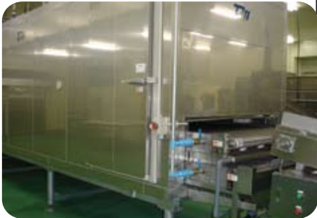
2-stage tunnel freezer
